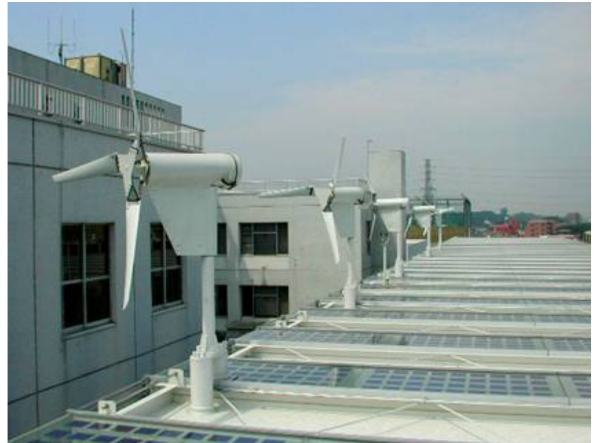
Small scale wind turbines and PVs on a rooftop
