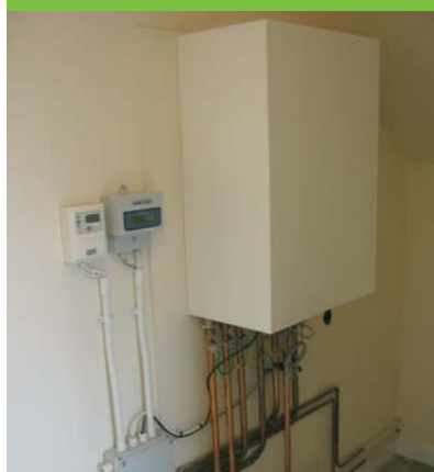
Example of a consumer interface unit without and with cover © Vital Energi
