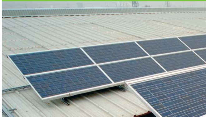
Building integrated photovoltaic panels and small-scale wind turbines
