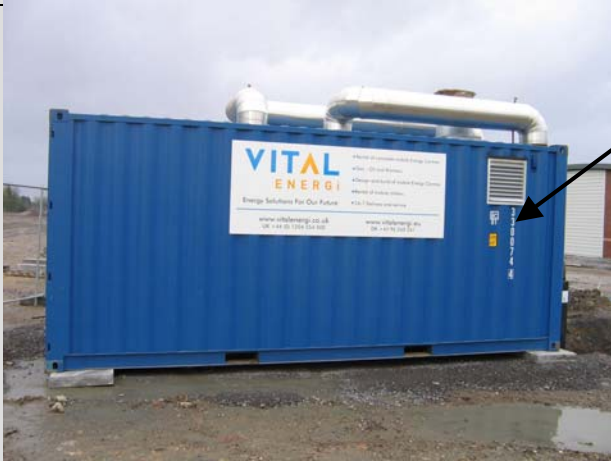
Temp. G-F boilerhouse
