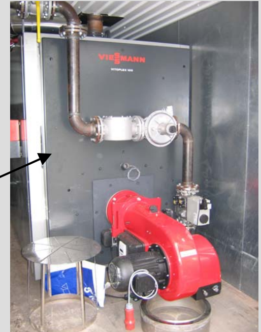
One MW boiler
