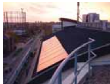
YHA Rotherhithe goes Solar with support from Renewable Energy Action for London. © YHA 2003
