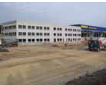
This distribution centre in Peterborough is heated and cooled by a ground sourced system. © Geoscience Ltd
