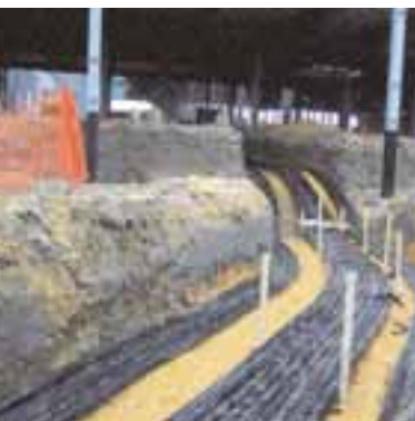
The offices at this distribution centre in Peterborough are heated and cooled by a ground source system.
