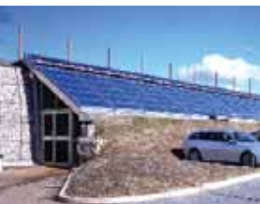
Solar power panels and solar heating at Renewable Energy System's head offices. © RES/Peter Mackinven
