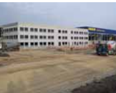
This distribution centre in Peterborough is heated and cooled by a ground sourced system. © Geoscience Ltd
