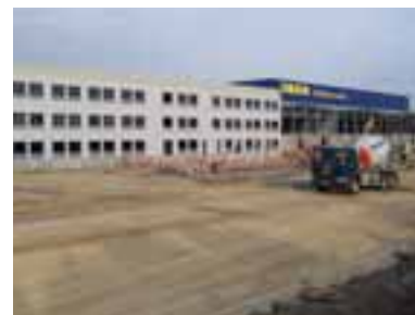
The offices at this distribution centre in Peterborough are heated and cooled by a ground source system. © Geoscience Ltd
