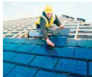
Solar power panels installed in the UK's first private commercial housing development in Edmonton, North London. © solarcentury
